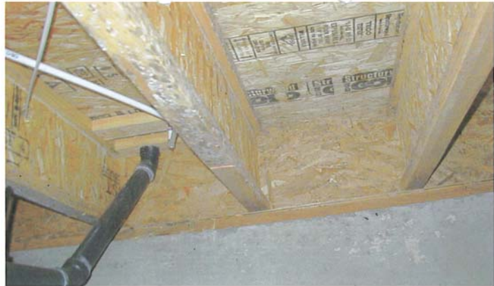
Proliferation of mold on the under floor of a residence in Sisters, Oregon
